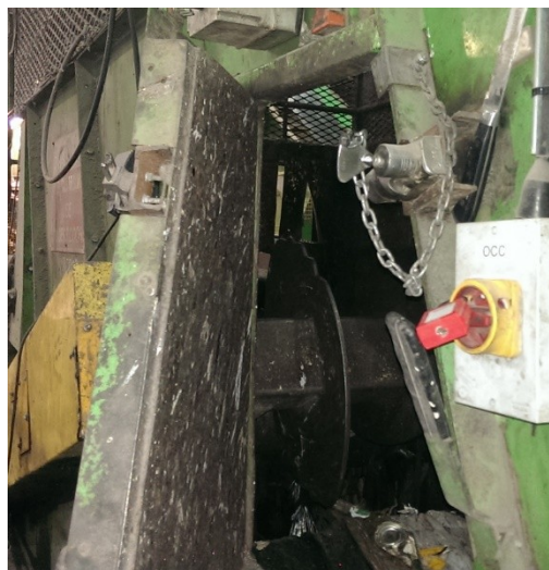
Access to the OCC for Maintenance & Cleaning
